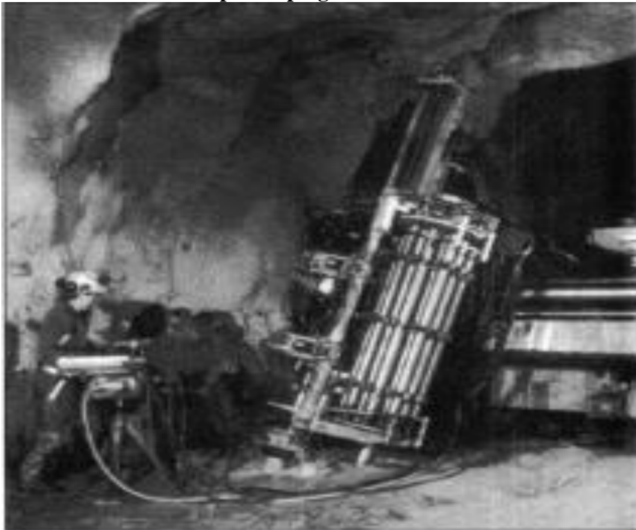
PICTURE 7. Longhole rig with slide positioning, remote control, and tube carousel Conclusions
